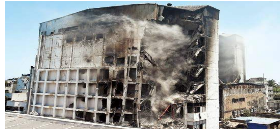
Fig: 2 Fire damaged buildings
