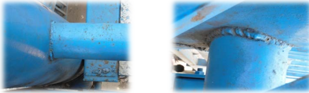
Fig 11: Welding connection we found at our site investigation.
