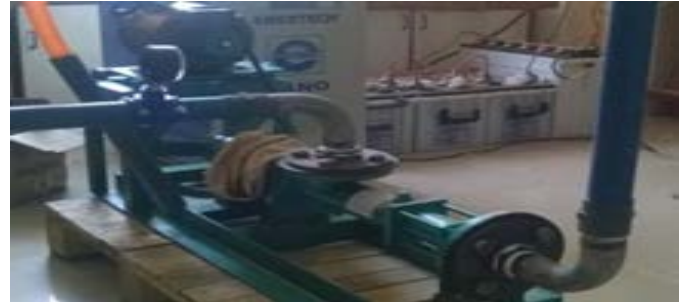
Fig -2: Solar power used for water pumping application
