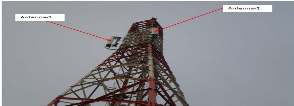
Figure 2: Snapshot of Tesebed mast with the Antennas: Base station CDMA 2000 1x
